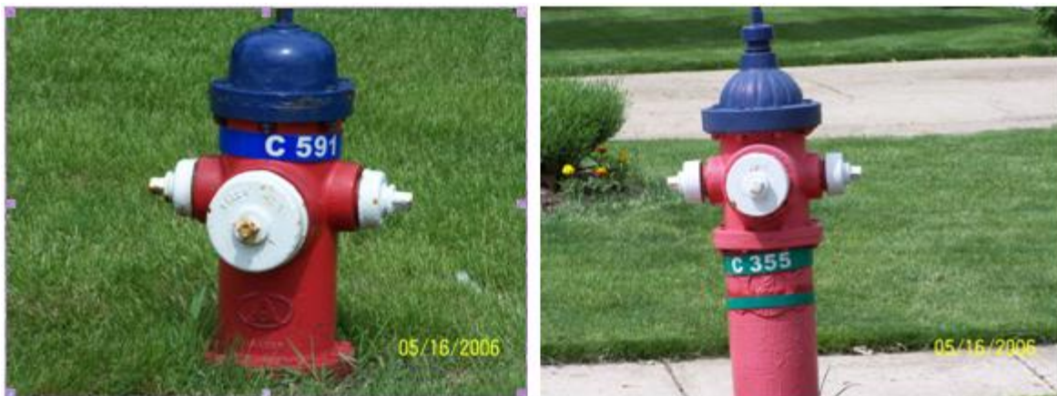
Figure 4 (a) Blue hydrant: > 1,500 gpm
